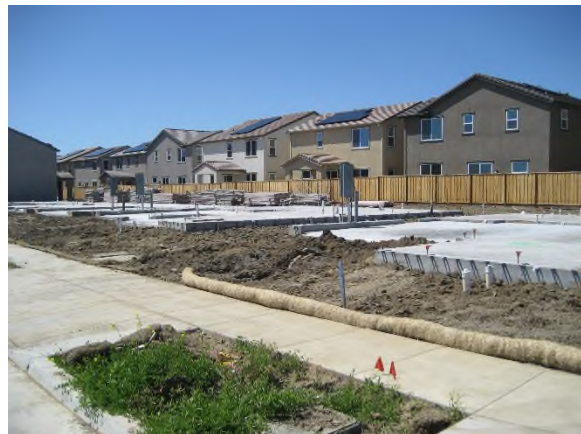
Homes under construction (foundations in foreground) and Substantially Completed homes (background) in Unit 4
