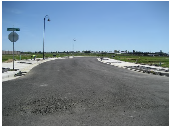
Looking south along Retreat Way in Unit 4 (final asphalt layer to be completed by Tri Pointe)
