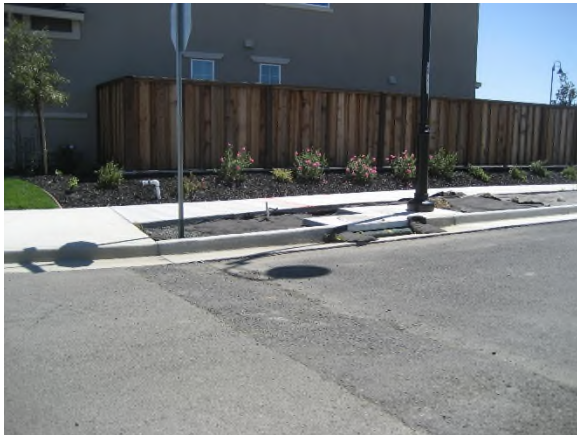
Final asphalt layer not yet completed west of Horizon Circle in Unit 4 (to be completed by Tri Pointe)
