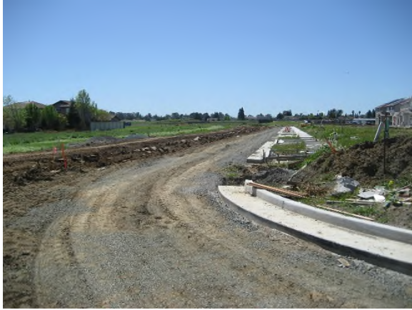
Looking southwest along Passion Ln. in Unit 4 (under development, an obligation of Tri Pointe)
